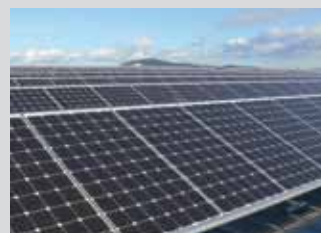
Gisinger Solarpark, Freiburg, 187 kWp
